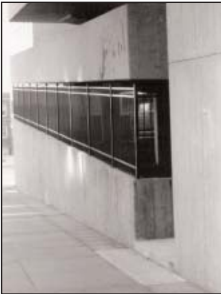
Use of mesh or grilles to block gaps between decks helps to reduce unauthorized access.
